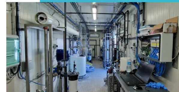
Above: Combinatory Pilot Plant in Venice Below: Nitrogen Recovery Pilot Plant
